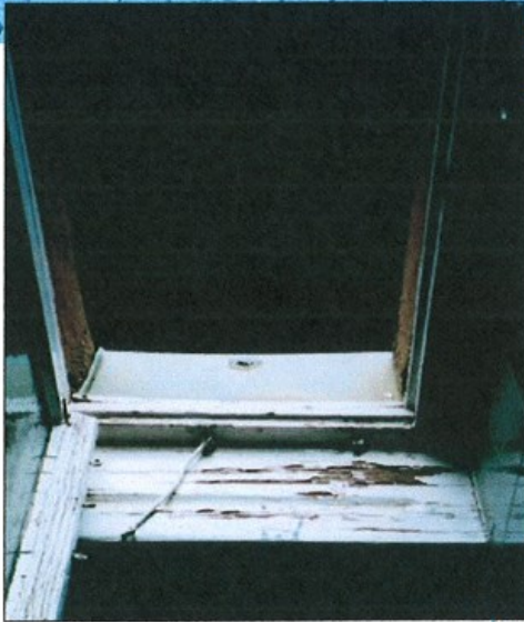
Leaky window – mold is beginning to rot the wooden frame and windowsill.
