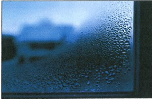
Condensation on the inside of a windowpane.
